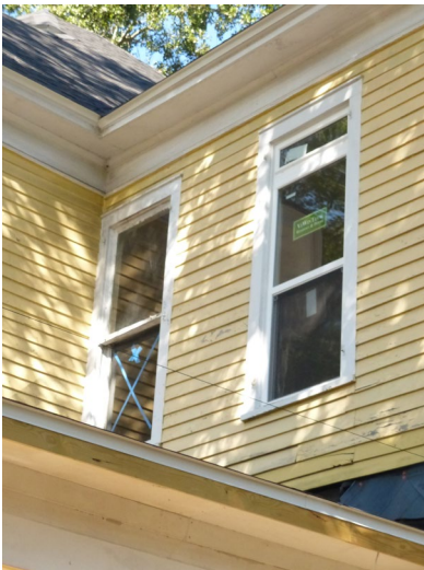
7. View northwest to east end of façade, 2 nd floor; original window at left; replacement window at right
