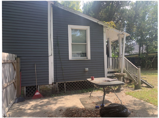
4. View of west end of north elevation (addition that replaced earlier rear projection)
