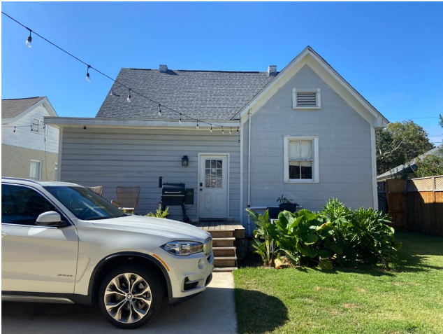
3. View of rear (east) elevation, looking west. Note fiber cement siding on flat roof portion and asbestos siding on gable cross-wing.
