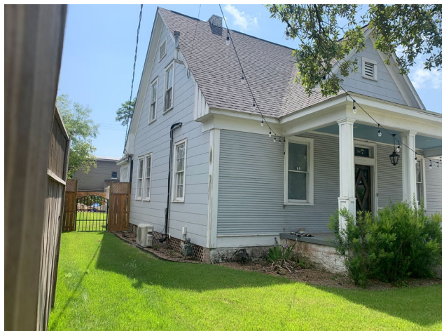
5. View of north elevation, looking southeast. Note mix of asbestos siding and wood drop siding.
