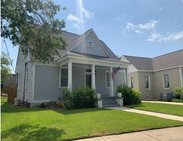
1. View of west façade, looking east. Note wood drop siding on façade and asbestos siding in center gable.
