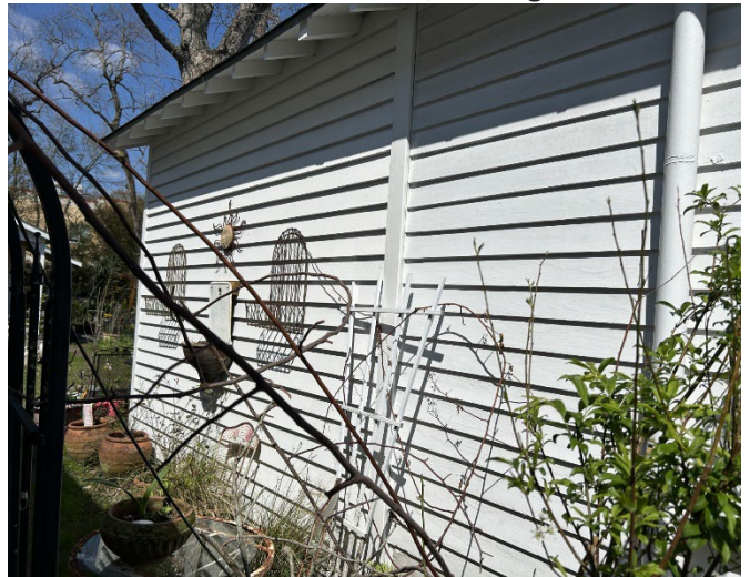
4. Detail of south elevation of addition, looking NW. Note retention of original corner board.
