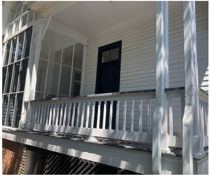
4. Existing door on southeast corner. Proposed new door for west side would match.
