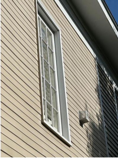
7. Detail of non-historic casement window on east elevation of rear addition, submitted by applicant
