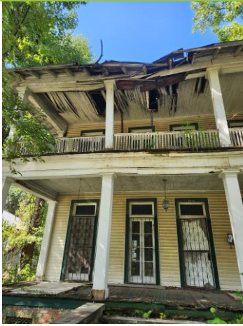
7. Detail of porch deterioration (submitted by applicant)
