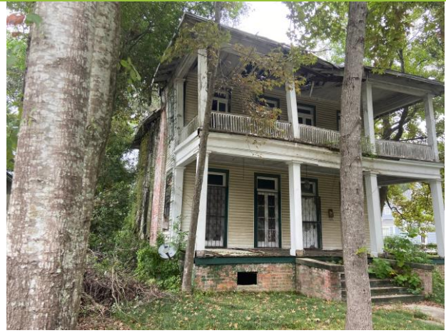
8. View of south façade and west wall. Note structural deterioration of west wall (submitted by applicant)
