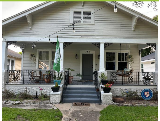
2. East façade, looking west. The four façade windows would be replaced with new wood sashes.
