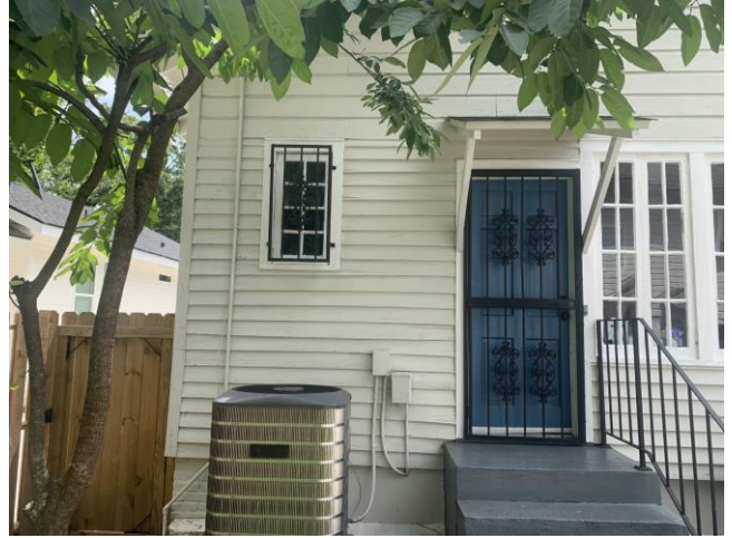
8. View of eight-lite fixed on west elevation. This window would remain. The two new eight-light windows proposed for the south end of the rear elevation would match this window.
